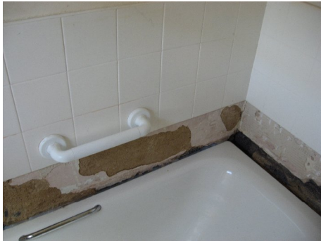
Swarcliffe: PFI contractors replaced existing bath with one that doesn't fit
